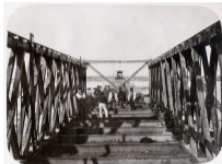
Framework of tube and staging no. 8, Victoria Bridge, Montreal, QC, 1859 , by William Notman. Collection of the McCord Stewart Museum, Montreal, Gift of Mr. James Geoffrey Notman (N-0000.193.127). Courtesy of the McCord Stewart Museum.
